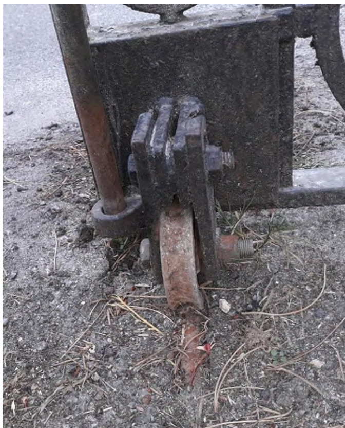
Figure 3- Gate supporting wheel (existing)
